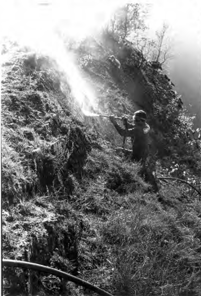
Wet sandblasting performed on a rock surface at Domkirkeodden, Hamar. Photo: Jon Markussen
